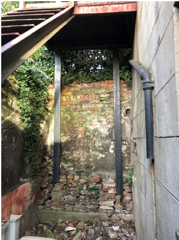
Existing stair structure to face of boundary partywall to 6 Westoe Village. Note, landing fixed to existing gable.
